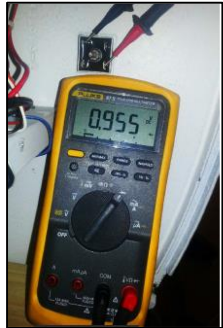
Above: Testing the Bridge Rectifier
